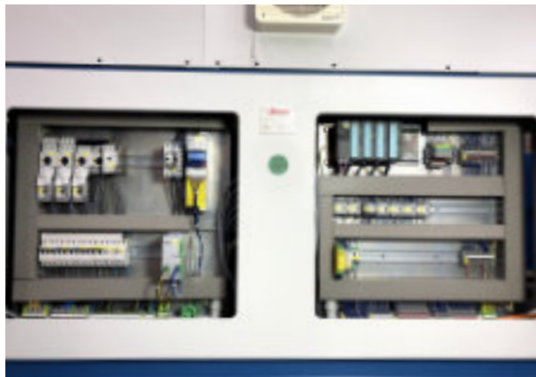
Electrical cabinet with remote maintenance
